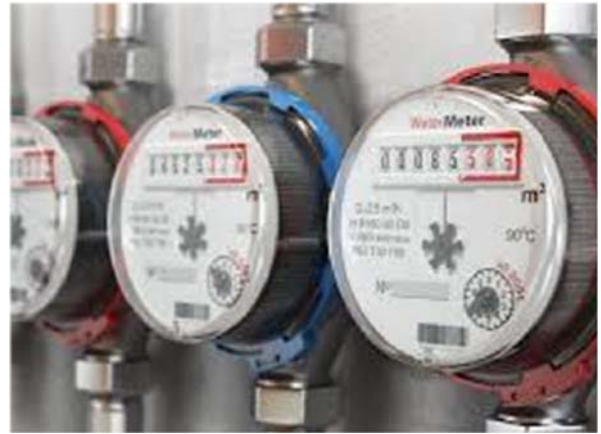
Water Metering systems
