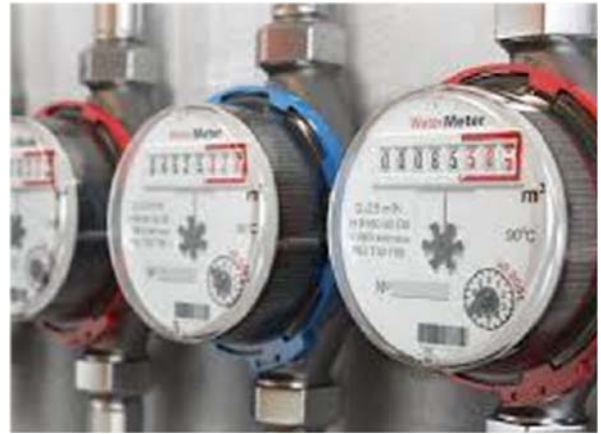
Water Metering systems
